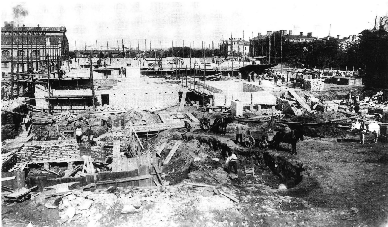
57. Work on the foundation of the theatre and concert-hall in Tallinn, 1911. Photograph by Parikas, ETM.
